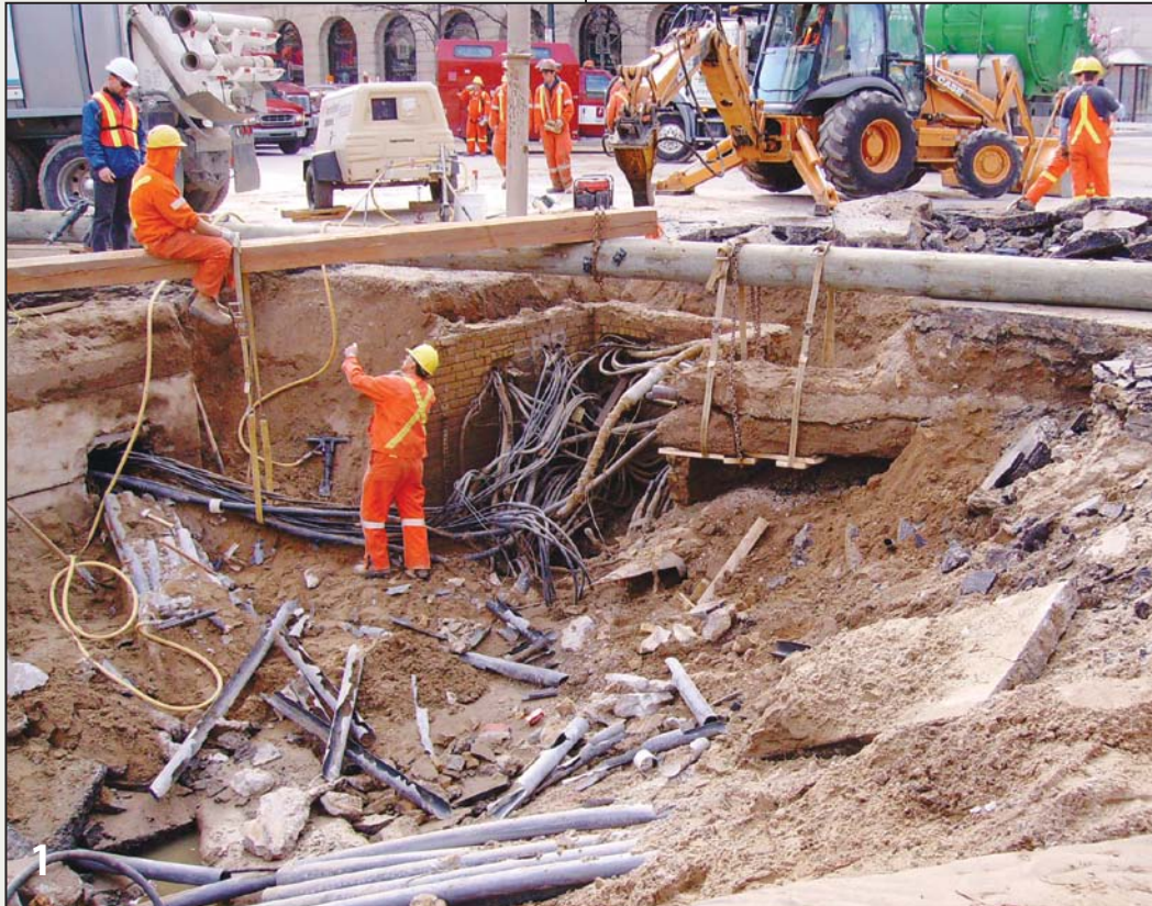
LONDON DISTRICT ENERGY
